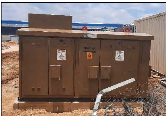
Phase 1: Central Hub - 500kVA miniature substation
