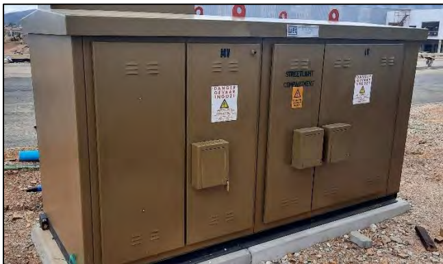
Phase 1: Gatehouse - 315kVA miniature substation
