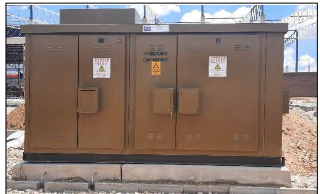
Phase 1: Hesto - 315kVA miniature substation
