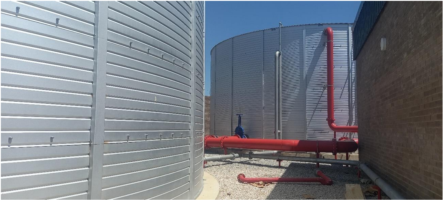
Fire Pump Station: Phase 1A
