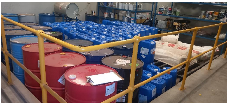
Feltex Building: Secluded Flammables Storage
