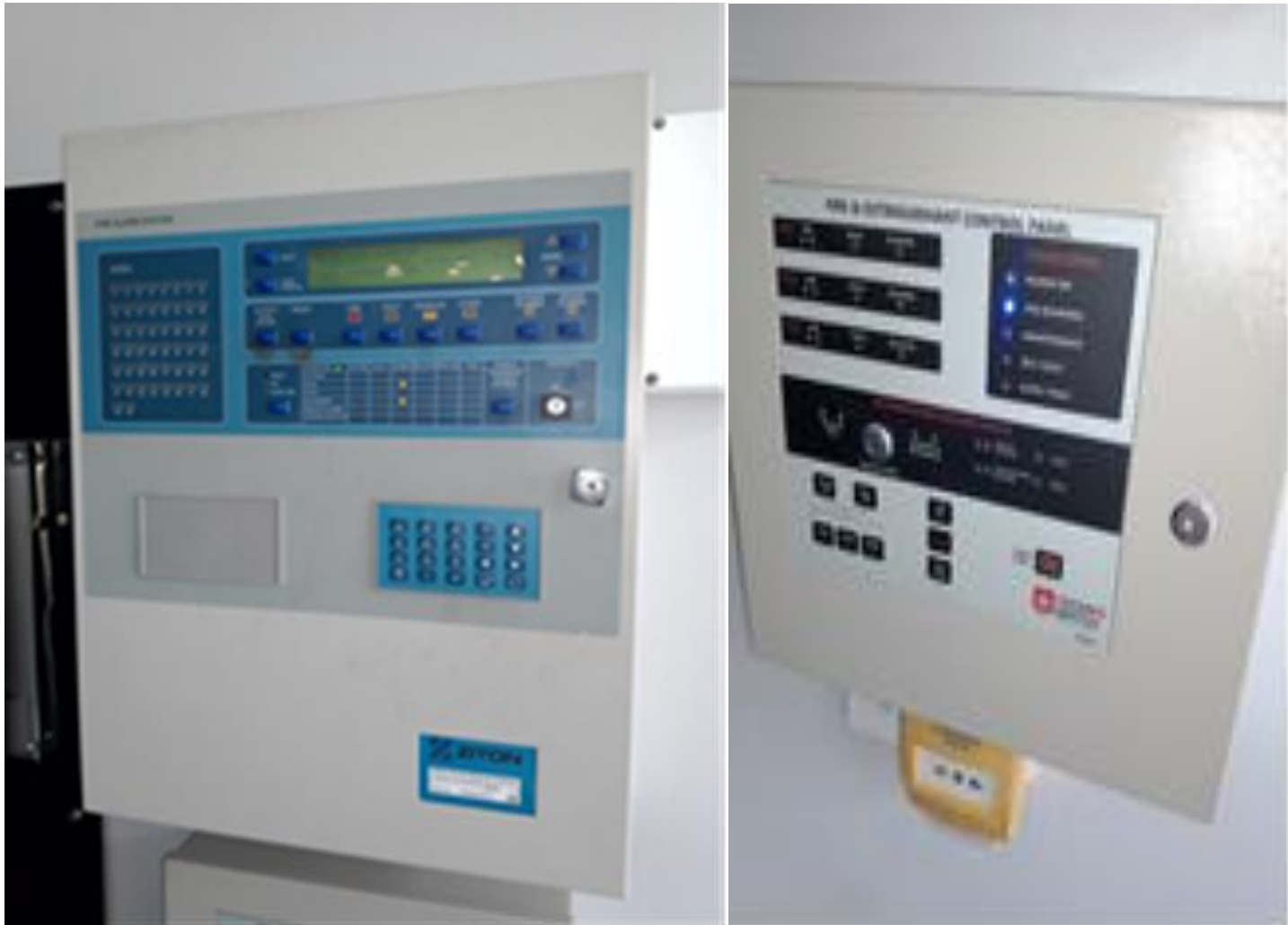
Feltex Building: Fire Panels (both detection and suppression systems) -All Zones Functioning Properly.
